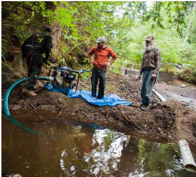
A backup diesel water pump is located beside the pool with the output hose draped over the dam. The water pump will be used to maintain full flow over the dam when the PVC pipe is temporarily removed to allow the excavator to remove sediment from that area.
