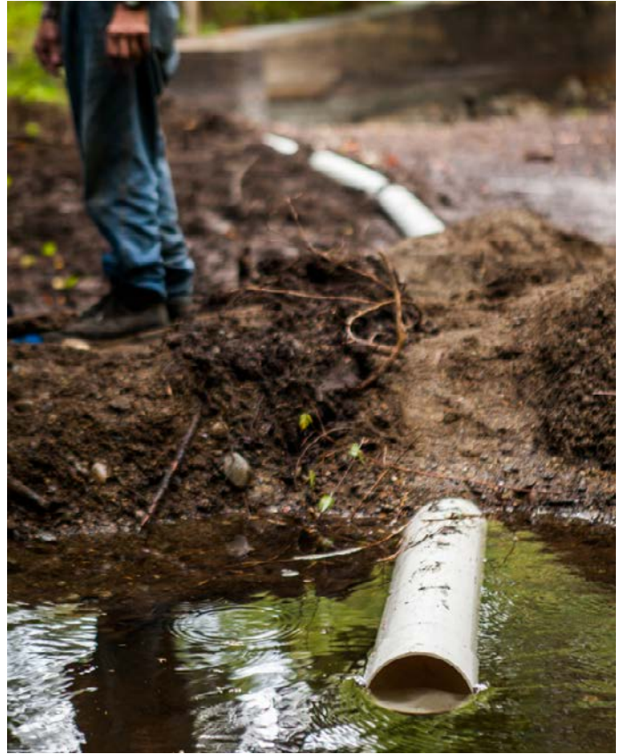
After fish are rescued from Carter Pond, the excavator digs a hole to create a pool where Terminal Creek enters Carter Pond. The 3 stop logs on the dam are removed one-at-a-time using ropes with hooks which attach to the hooks on the stop logs. For safety reasons, BIFWC volunteers are careful not to create sudden heavy surges of water over the dam into Terminal Creek downstream. A 6" PVC sectional pipe gravity feeds clear water from the pool over the dam where the stop logs used to be located. Note that only 1 stop log remains (soon to be removed completely) and it has been lifted slightly to allow the water to drain slowly; the same procedure was followed with the top 2 stop logs.
