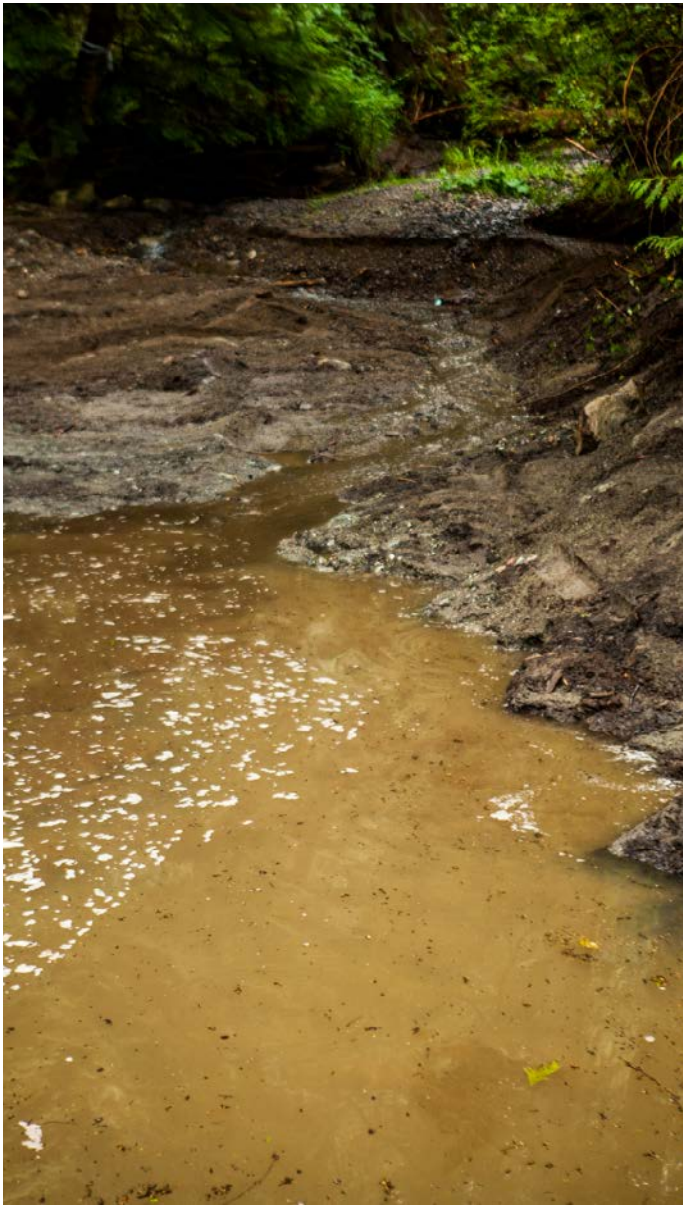
When all sediment has been removed, the pool at the entrance to Carter Pond is released and the PVC pipe removed. The pond refills and water soon flows over the dam.
