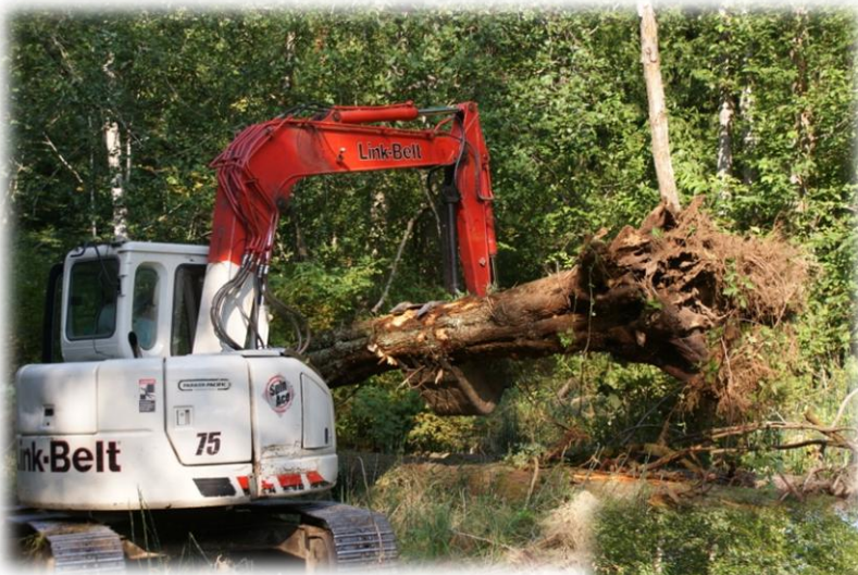
Windfalls were removed from beside Davies Creek close to Dorman Road in Crippen Regional Park. Access was gained from the "lower ball field."
